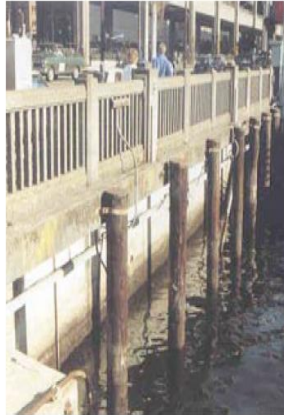
Fender piles require protection against marine borers and need high wear resistance.
